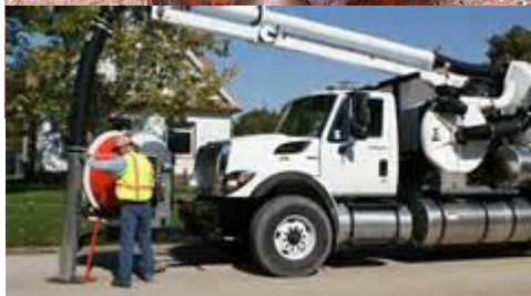
The high pressure water moves the jetter head through the sewer line while vacuum on the truck pulls up dislodged debris.
